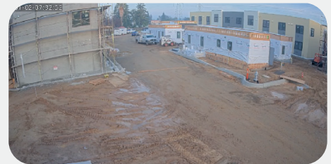
Multiple Cameras for Multi-direction Visibility and Perimeter Coverage
